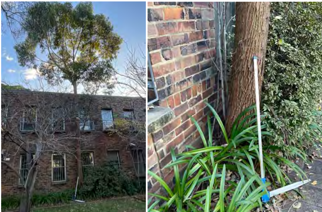
Figures 28 & 29: Tree 25 in the landscape (Left) and its very close proximity to the existing wall (Right). (Source: Fisher 23 rd June 2022).
