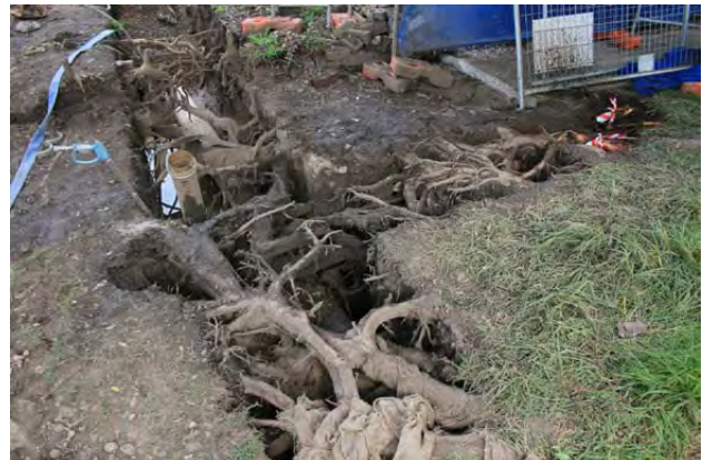
Figure 96- Non-destructive excavation methods can allow services to be installed across verges without the need to sever important and structural tree roots. (Photo: Arterra)
